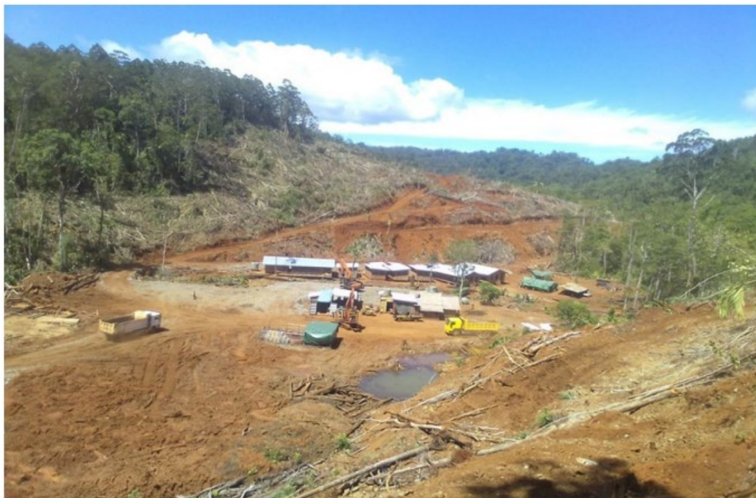
Photo 2: Construction of mining contractor area in foreground opposite 50man camp. Commencement of haul road construction in background.
